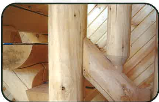
← Bevel Cut A bevel cut is made on both sides of the top and bottom rail before attaching to the posts.
